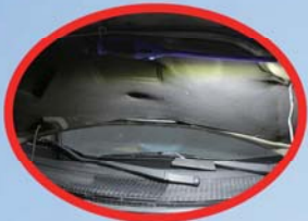
Engine room lighting
